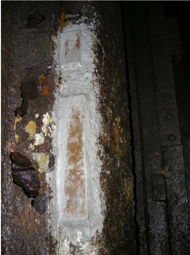
Damaged spot straight after coating with MM-metal UW
