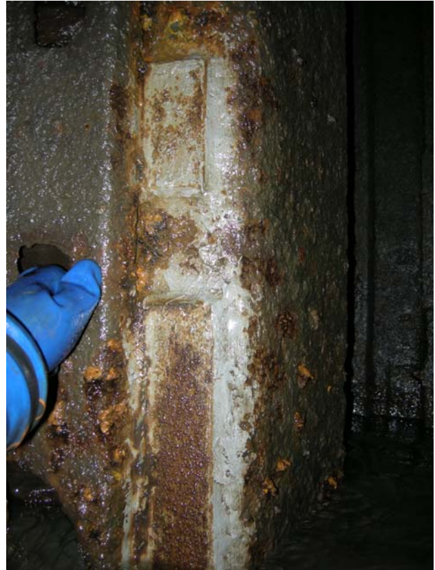
Damaged spot approx. one year later
